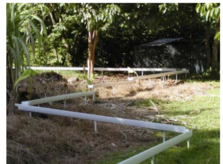
Effluent irrigation system.
