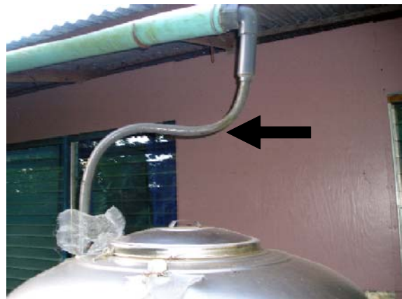
The arrow points to an area in the piping that allows water to stagnate, resulting in bacteria growth and poor water quality.
