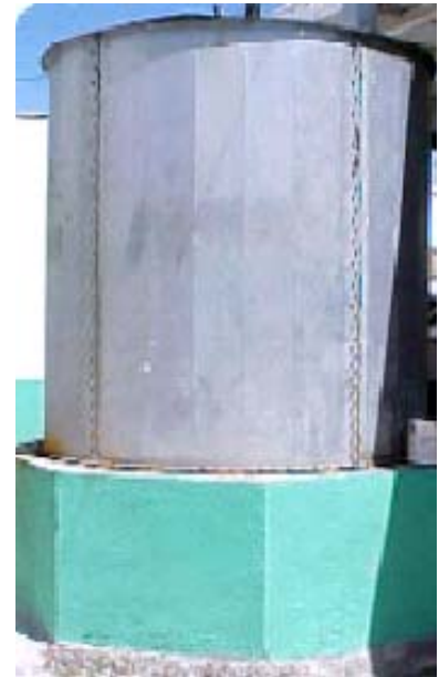
This concrete foundation is appropriate because it keeps the tank level.
