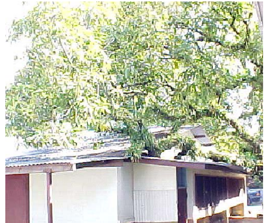
Trim tree branches to avoid giving rats, cats, and lizards access to your roof.
