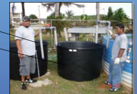
Plastic tank (400 gallon) and 2" siphon tubes
