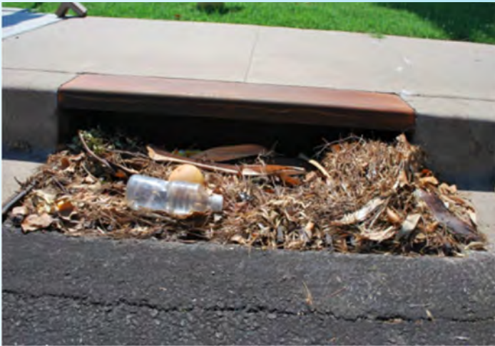
Figure 8. Storm Drain Clogged with Litter and Debris
