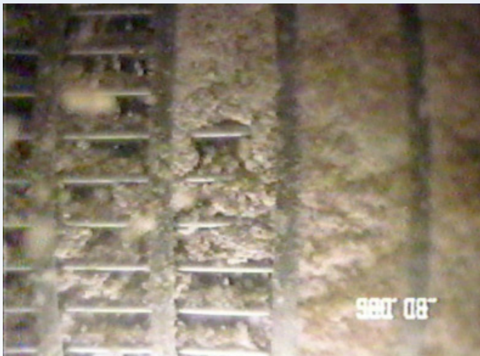
Figure 2: Scale formation on well screen.
