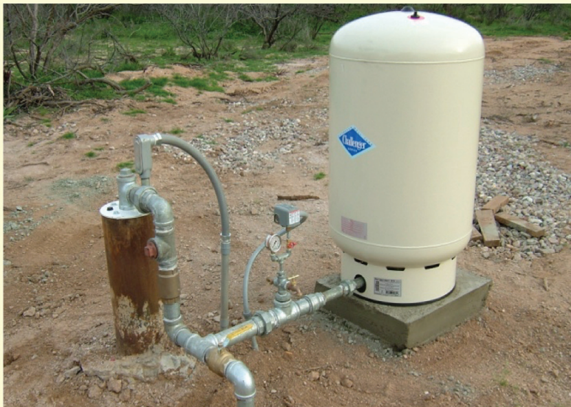
Figure 1. Example of well casing, pressure switch and pressure tank in Arizona. photo: G. Hix.
