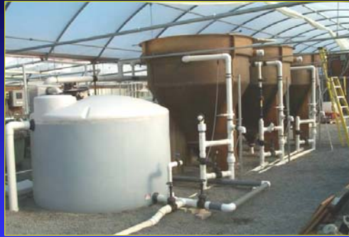
Off-line Settling Tanks at Freshwater Institute
