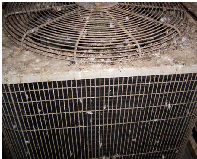
Air exchange unit covered in pigeon excrement
