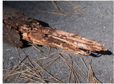
Desert dampwood termite damage to post Photo: USDA-FS
