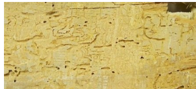
Powderpost beetle damage below surface Photo: Western Australia Dept. of Ag.
