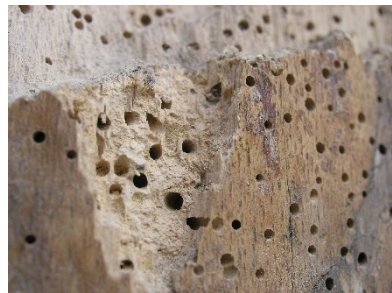
Deathwatch beetle exit holes in wood. Note uneven sizes of holes. Photo: Kai-Martin Knaak
