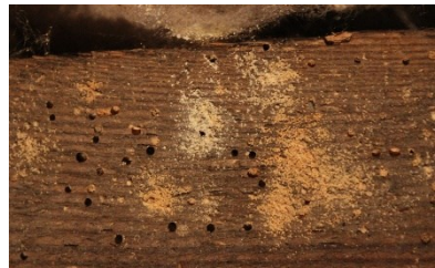
Powderpost beetle damage Photo: InArc Design, www.inarc.ie
