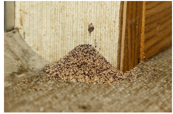
Sign of western drywood termite damage Photo: Kevin (fbkev2002)
