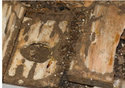
Pacific dampwood termite damage. Photo: Kevin Lentz
