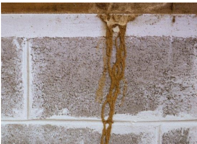
Subterranean termite-working tubes Photo: USDA-Forest Service
