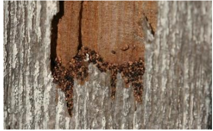
Western drywood termite damage Photo: Whitney Cranshaw
