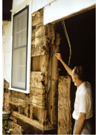
Extensive damage to wooden structure by subterranean termites Photo: USDA Forest Service
