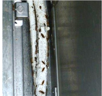
German cockroaches along and behind electric cables Photo: Armed Forces Pest Management Board
