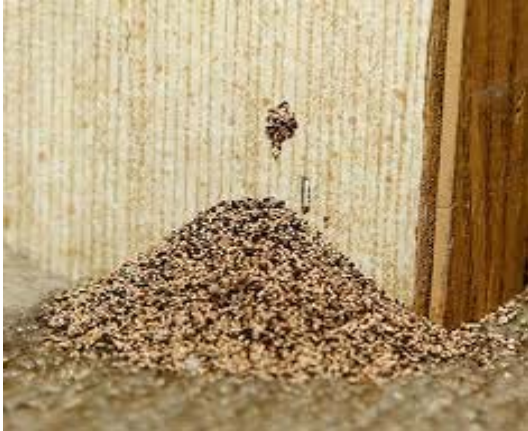
Sign of western drywood termite damage Photo: Kevin (ibkev2002)
