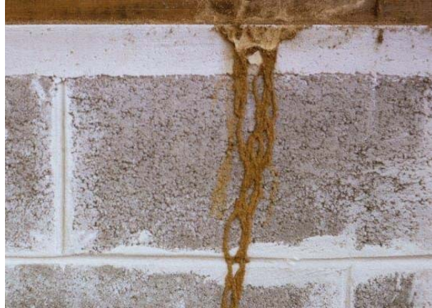
Subterranean termite-working tubes Photo: USDA-Forest Service
