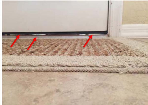
This locked door is wide open to pests! See light coming in through gaps under door. Photo: Dawn Gouge
