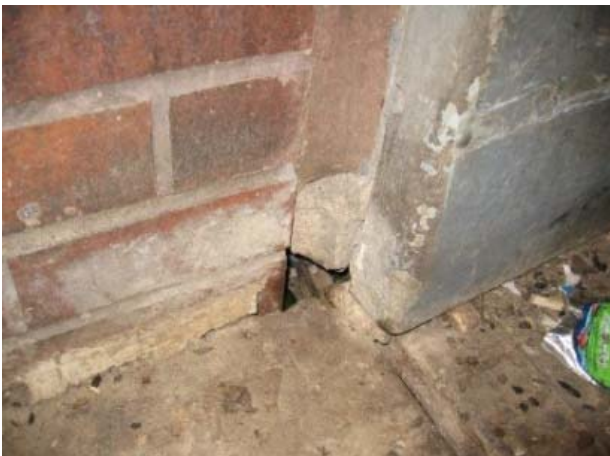
Gaps or holes in walls or foundations provide entryways to rats. Photo: Dawn Gouge
