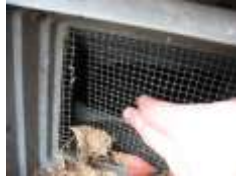
Torn mesh on drain cover must be reported
