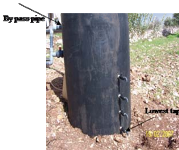
Figure 4. Photo showing the AC with the taps and by pass pipe
