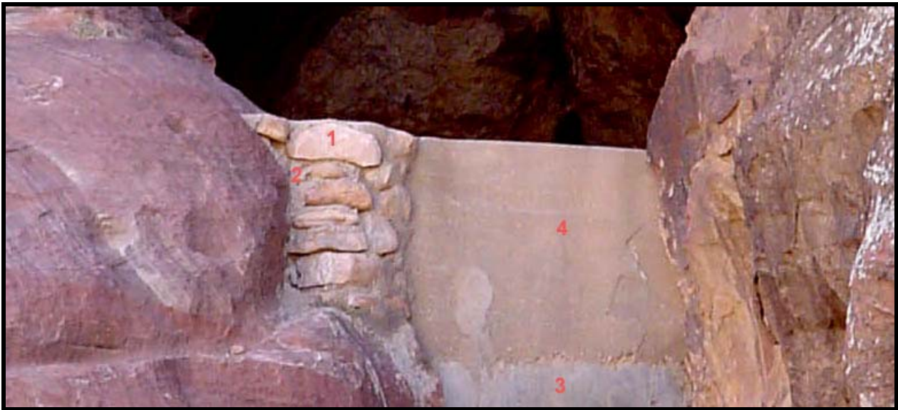
Figure 8: Here we see at least four periods of reconstruction on the Ba'aja dam -- an excellent venue for interpretive material on the history of water conservation.
